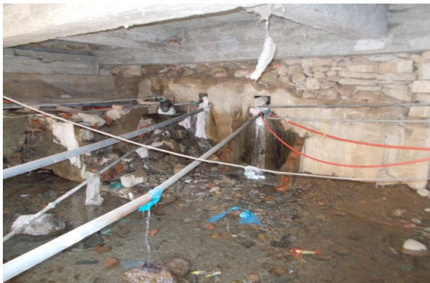
Piped Water supply network from natural spring-Banihal
